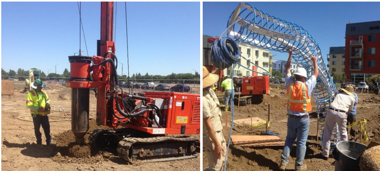
Figure 4. (Left) Drilling rig boring holes for GHEs. (Right) Lowering helix coil for dry bore in ground.
